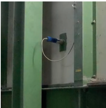
INSTALLATION ON A CHUTE FOR MIN LEVEL DETECTION
