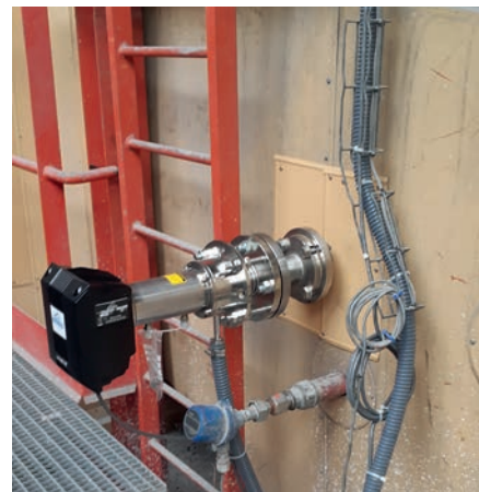
CROSS DUCT, INLINE COMBUSTION MONITORING
